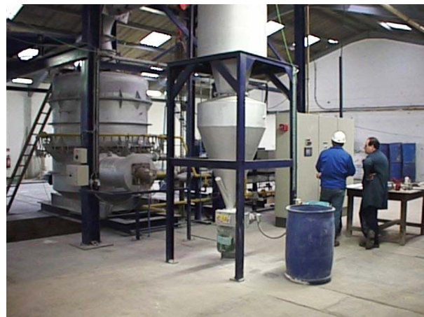
High Temperature Mineral Calciner
